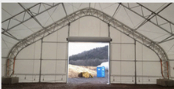
RES, Ballast Anchoring System in Scranton PA
