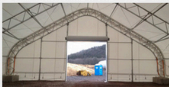
RES, Ballast Anchoring System in Scranton PA
